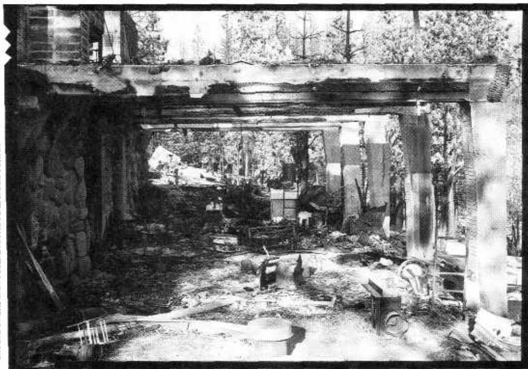
The burnt out shell of the Gunderson home.
