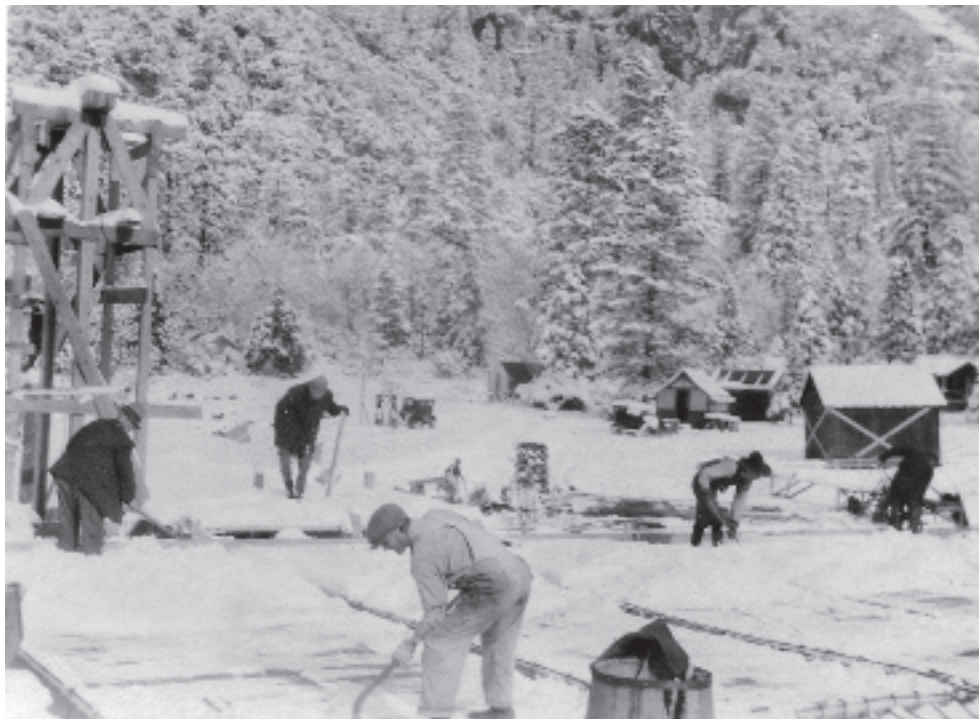
Workers toiled through the winter of 1924 to build the Museum. Here, workers shovel snow from the building's floor slab forms so they can continue construction.
