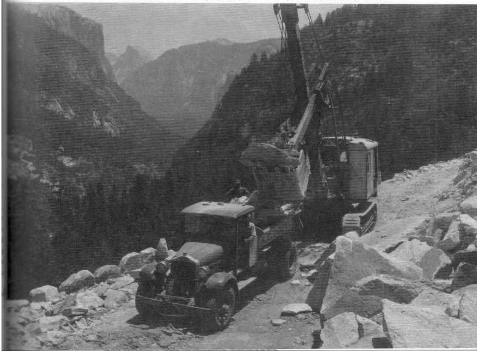
Contractor's truck and steam shovel at work clearing rocks from the right-of-way on the western approach to the Wawona Tunnel.
